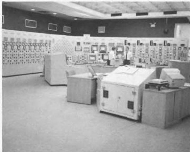
47. Production without people: Dungeness nuclear power station.
